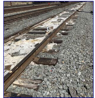
Traditional Mat, UV degraded 6 months After Installation.
