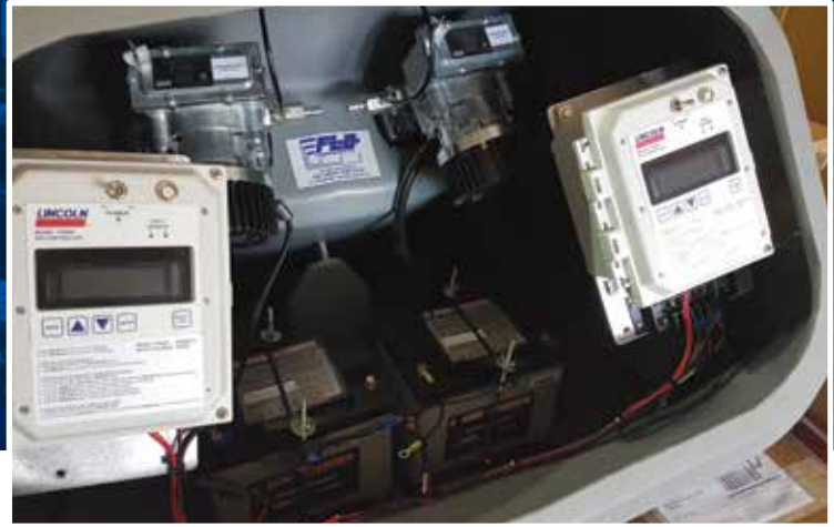
Solar powered stationary or wayside rail lubrication systems lower noise emission and reduce wear on rails, switches and wheels. This controller can transmit and receive system information on any hand-held device.
